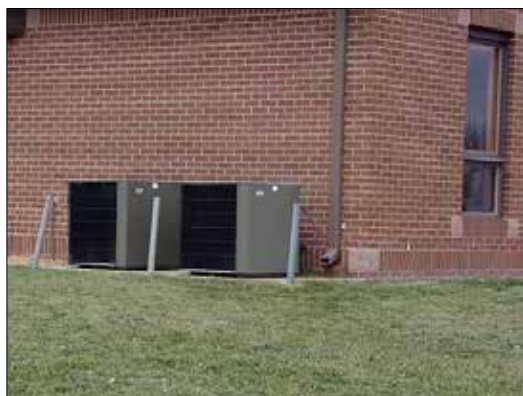
Example: This photograph illustrates AC units located at the back of the building creating an easy target for theft.
