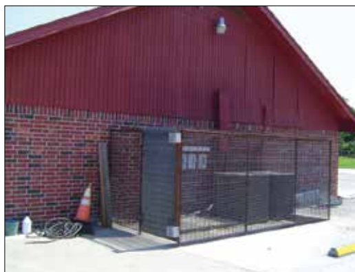
Example: This photograph illustrates AC units protected by a steel cage and security lighting.
